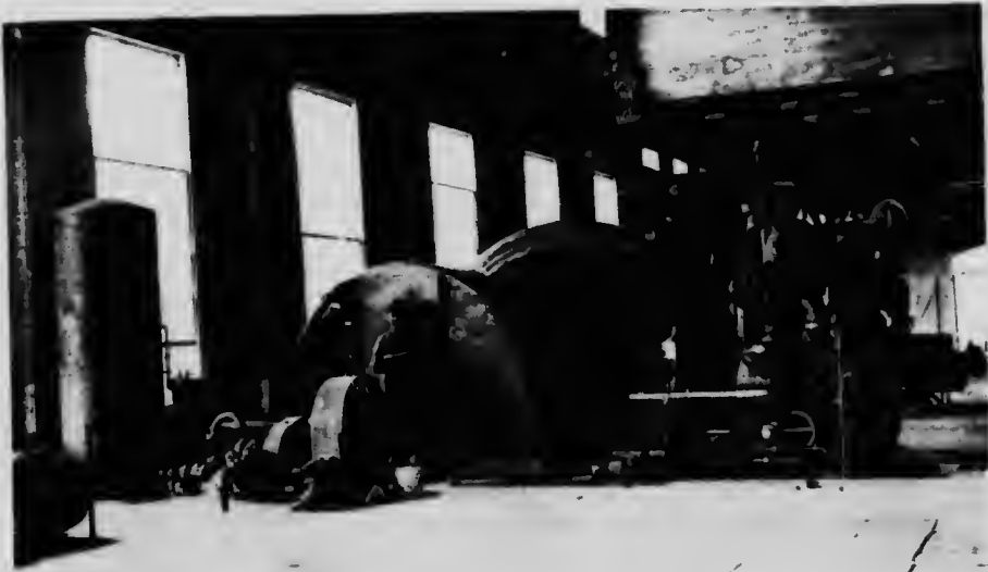
Vancouver Island Power Company Limited. No. 3 unit in position showing governors, oil pumps and gate valves.
